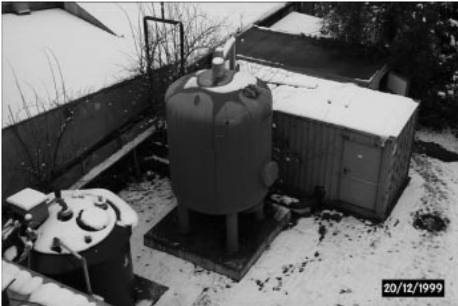
Groundwater Remediation Unit (in wintertime)
