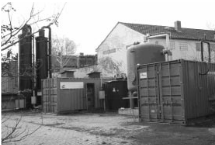
Groundwater Remediation Plant
